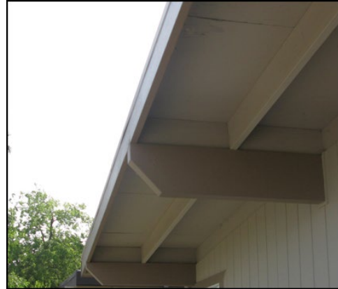
(Beam cut at an angle)
