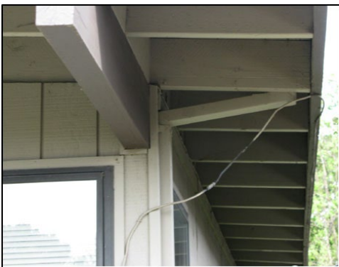
(Drooping cable line)
