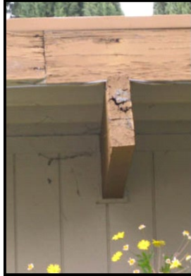
(Beam and fascia with dry rot and sun damage)
